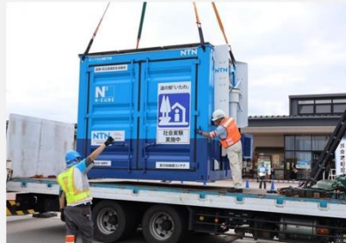
Demonstration test held at the roadside station "Itano" which is one of the "disaster prevention roadside stations" selected by the Ministry of Land, Infrastructure, Transport and Tourism (September 2024)
