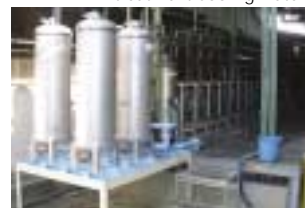
Reusing rainwater as heat treatment cooling water
