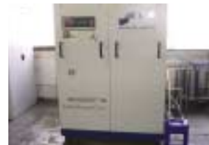
Vacuum distillation unit
