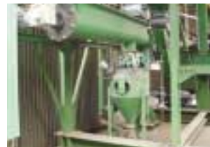
Waste sand pneumatic transfer unit
