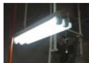
Fluorescent light with pull switch
